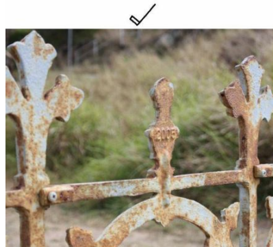
Figure SC6.3.5.36 Illustrates an example of a desirable outcome - date stamp on new or introduced fencing panel
